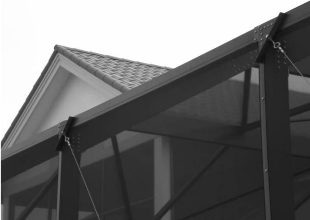
Approved cable set connections
